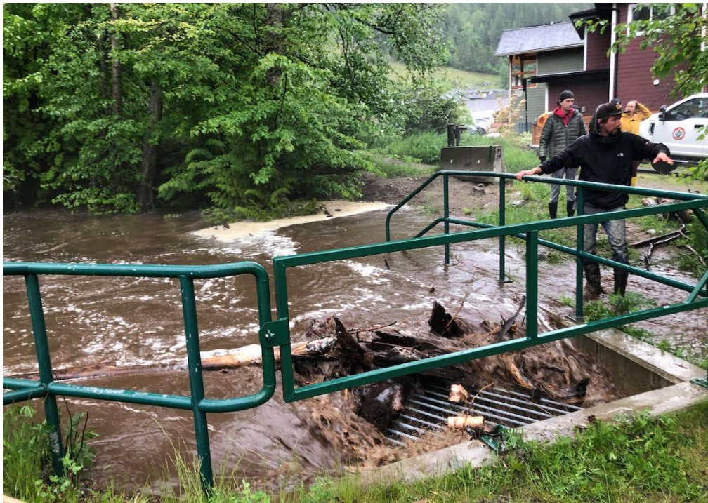
Figure 3-6. Overflowing culvert at Anderson Creek (June 2nd, 2020, Photo: Nelson Star)
