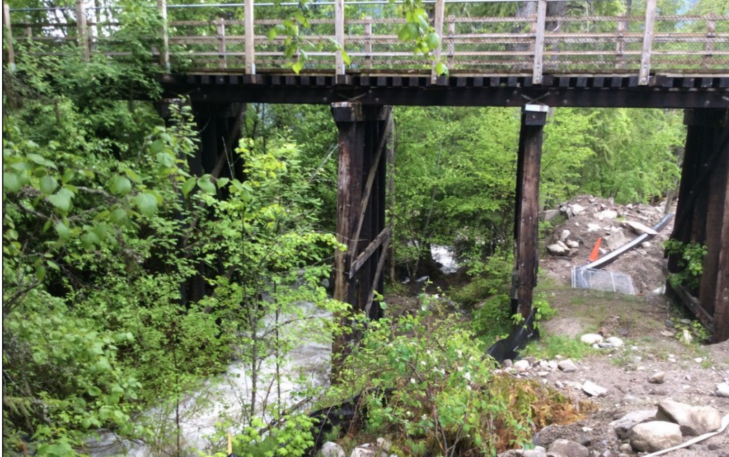
Figure 3-2. Trestle bridge over Anderson Creek near the fan apex. Wooden trestles would likely suffer major damage during a debris flood. Photo: BGC, June 12, 2022.
