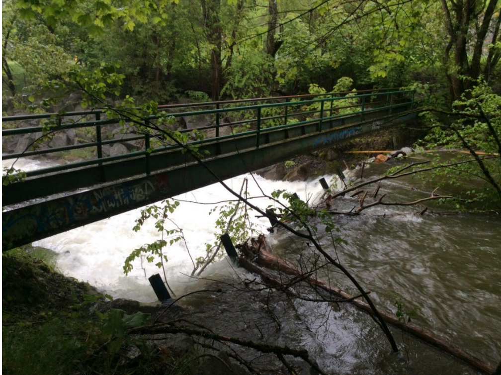
Figure 3-12. Debris barrier across Cottonwood Creek approximately 60 m upstream of culvert below Highway 6. Photo: BGC, June 12, 2022.
