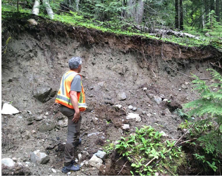
Figure 3-9. Till exposure along a property access road at approximately elevation 820 m near the Ward Creek drainage. Photo: BGC, June 12, 2022.
