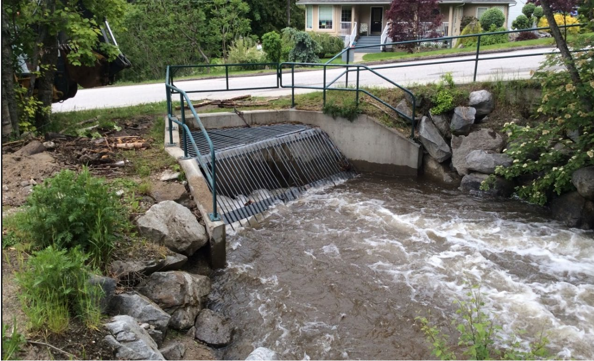
Figure 3-5. High flows at the upper culvert on Elway Drive with an engineered trash rack to avoid organic debris and large boulders from entering the culvert. Photo: BGC, June 12, 2022.
